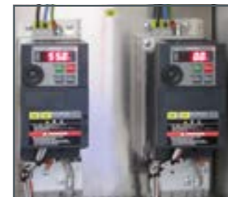
Frequency converters for controlling the pumps
