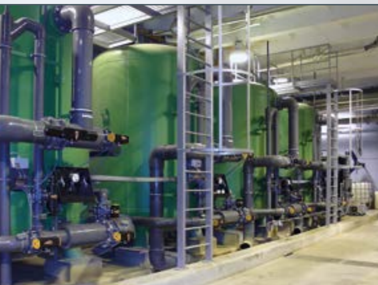
Continuous-flow adsorber in a water treatment plant
