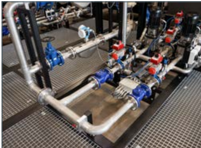
Field process: redundant pumps and Coriolis flowmeters
