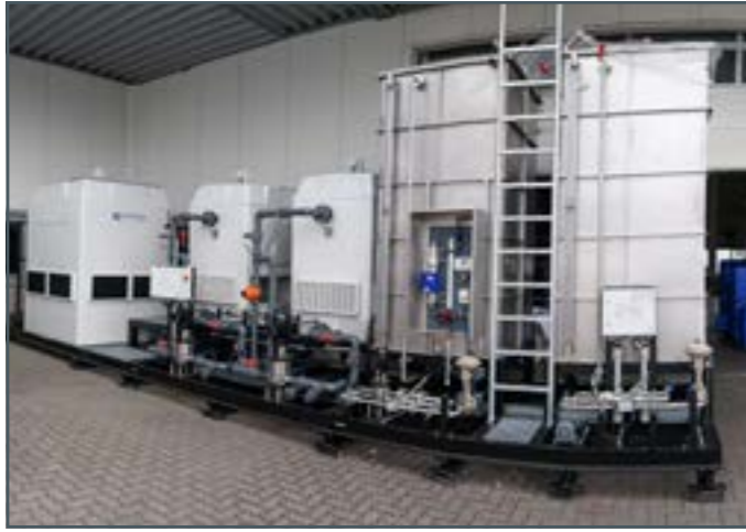
Outdoor wet cooling towers and receiving tanks for process water and ethylene glycol
