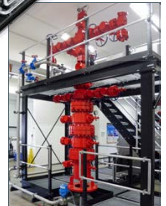
Wellhead and Xmas-tree
