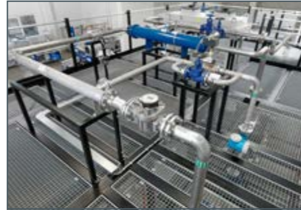
Thermal reactor with chemical injection system
