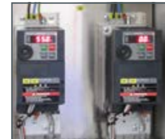
Frequency converters for controlling the pumps
