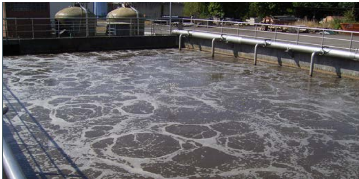
Biological treatment stage on a wastewater treatment plant (aeration tank)
