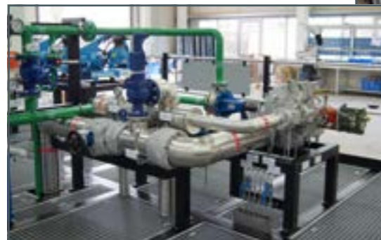
Steam driven auxiliary pumping station
