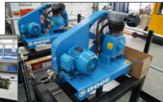
Compressed air station
