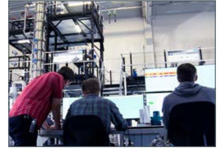
IPP during test operation before delivery of the plant
