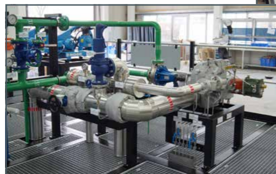
Steam driven auxiliary pumping station
