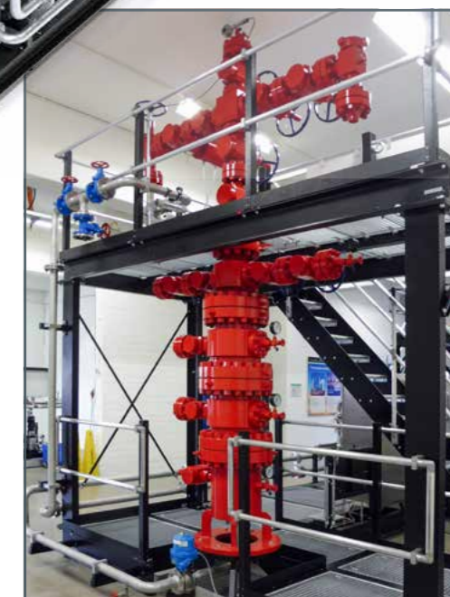
Wellhead and Xmas-tree
