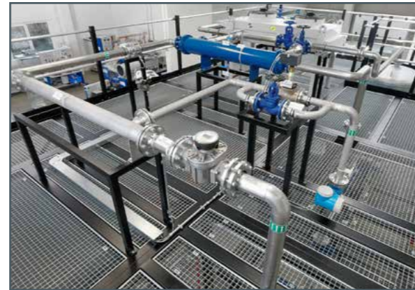
Thermal reactor with chemical injection system
