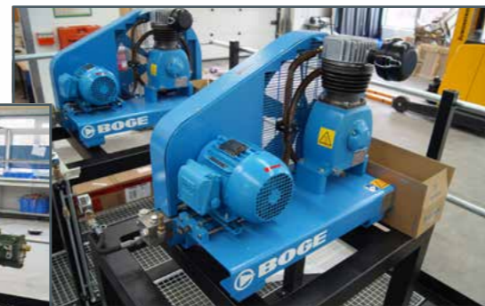
Compressed air station
