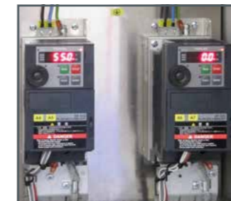
Frequency converters for controlling the pumps
